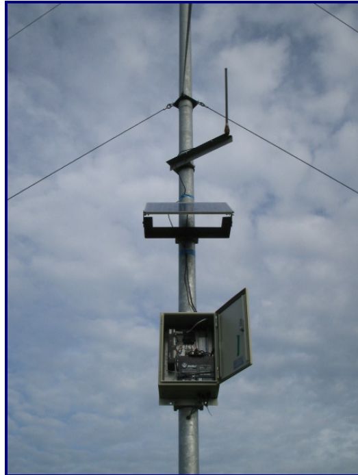
Instrument Enclosure in Good Condition
