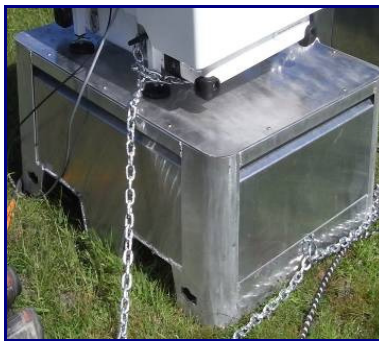
Fig 3 - Secondary Battery Storage unit:
